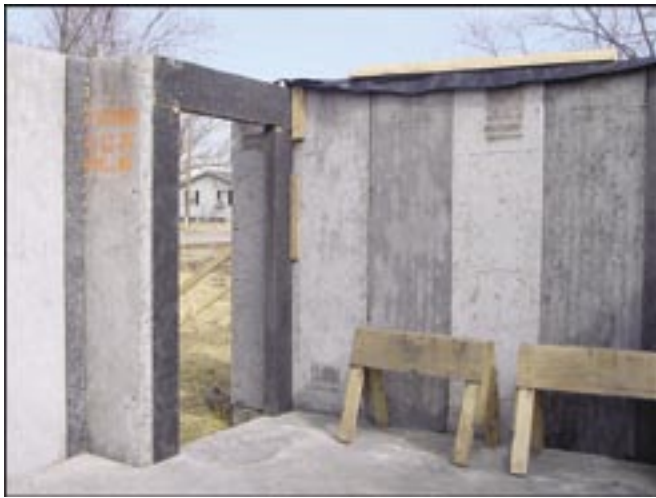
Eight foot high panels are locked together solidly to form insulated, windproof, quake proof and fire proof walls in home under construction.
